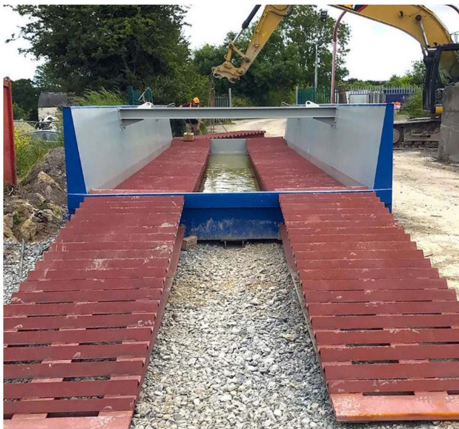
Plate 3-1: Example of self-contained wheel wash system. Source: https://www.glanaco.ie/product/wheel-wash-bath-system/
